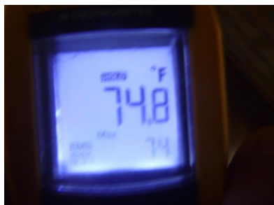
10.0.B Item 1 (Picture) Return Air Temp
